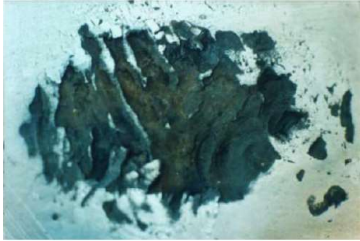
Figura 51: Foto de defecto shelling, [30].
