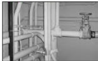
Piping and plumbing systems Photo by John M. Cimbal.
